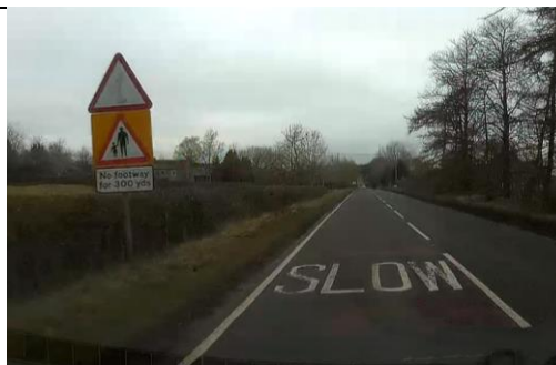
Photo 17 - Warning sign face is badly worn and requires replacement
