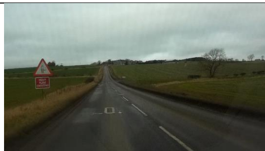
Photo 12 - Example of worn sign and SLOW road markings which can be improved.
