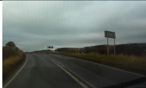
Photo 6- Example of location where enhanced chevron signing on bend may be beneficial along with road marking/stud refreshment.
