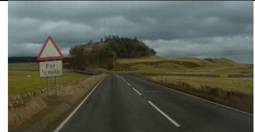
Photo 26 – Badly worn double bend warning sign. Sign and supplementary plate could be enhanced on yellow backing board
