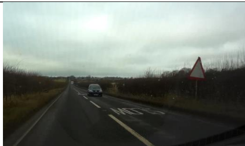
Photo 15 – Warning sign face is badly worn and requires replacement and sign is twisted to face in the wrong direction.
