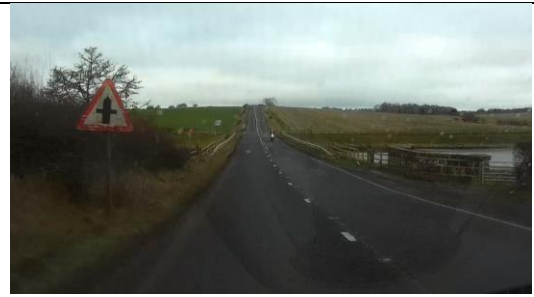
Photo 14 - Worn junction warning sign which can be improved and opportunity to provide SLOW road markings and red strips.
