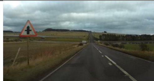
Photo 32 - Example of crossroads warning sign which could be enhanced on yellow backing board with a supplementary distance plate
