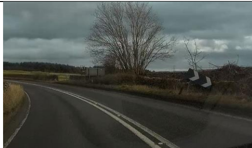
Photo 27 – Chevron sign has been dislodged and is facing the wrong way – should be directing traffic left around the bend.
