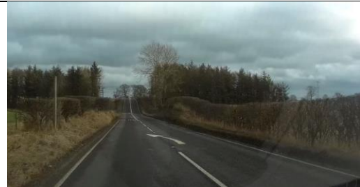
Photo 24 – Missing warning sign (vacant post) in advance of a section of road with non standard vertical and horizontal alignment.
